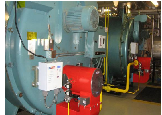
After Mark-6 Controller and EGA
