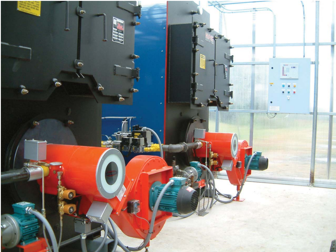
Limpsfield LC9 dual fuel burners on Hurst boilers
