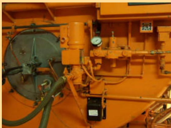
Existing burner/boiler Setup prior to retrofit
